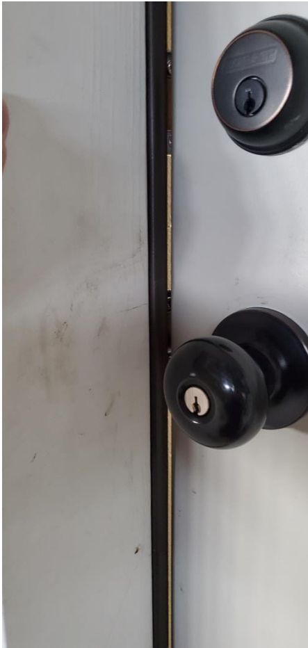
Door is fully closed but there is still a gap
