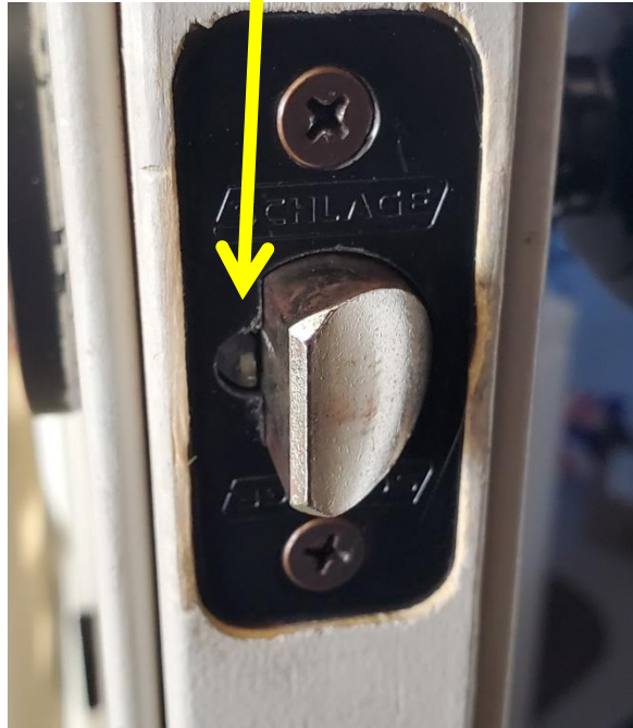
Latch pin is broken off
